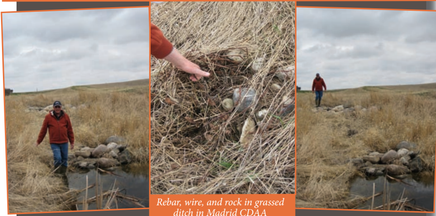
Elevation changes in a flax bale and rock drop structure in Madrid CDAA
